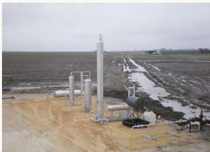
Figure 4 – processing facilities at the Smith #1 well site
