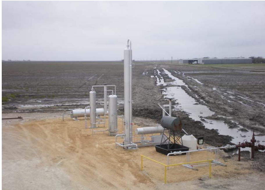
Figure 4 – processing facilities at the Smith #1 well site
